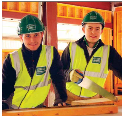
Christopher Kerr (left) and Sean Karte, working on the multi-million pound accommodation project at the University of Stirling.
